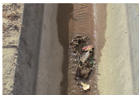
Note: Garbage clogging misclassified as silt clogging, with a confidence score of 0.5490 for the silt category.
