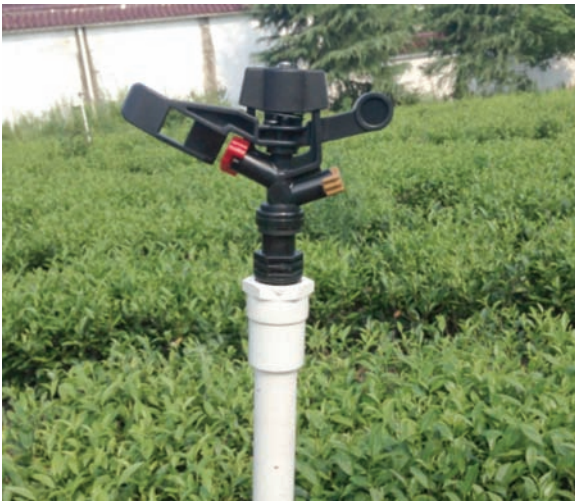
Figure 2 Frost protection sprinkler
