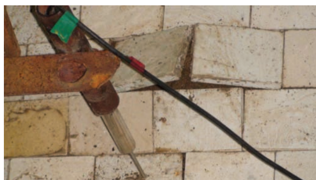
Figure 7 Uneven frost damage phenomena
