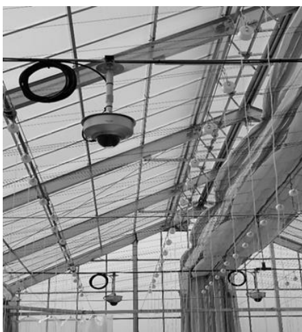
Figure 9 Three network cameras are strategically installed in a bay for monitoring of the crop growth
